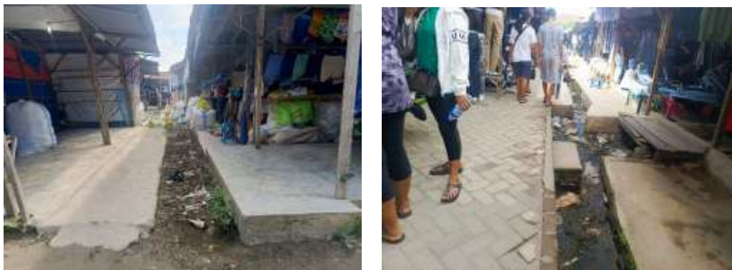
Picture 2 Infrastructure Degradation and Sanitation Crisis in pajak melati
